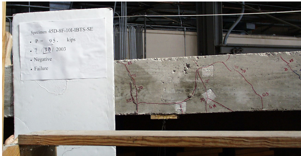
Figure 5-14 Interior bay failure surface at side of slab, facing north
