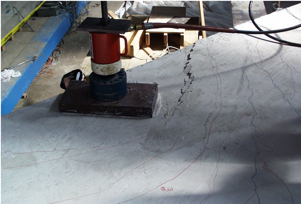
Figure 5-25 Interior bay failure surface at top of slab, facing north
