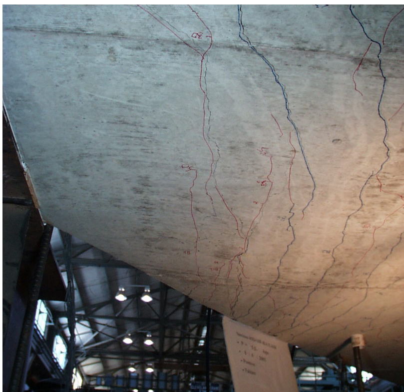
Figure 5-50 Failure surface at bottom of slab, facing north
