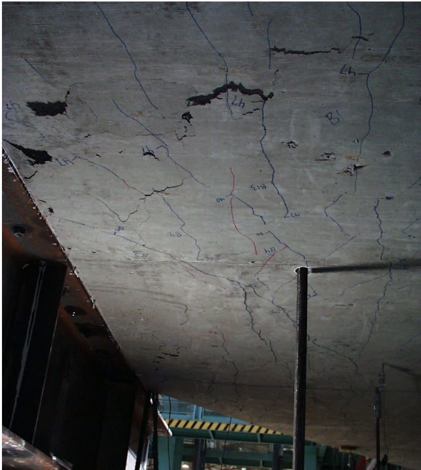
Figure 5-30 Exterior bay failure at bottom of slab, facing north
