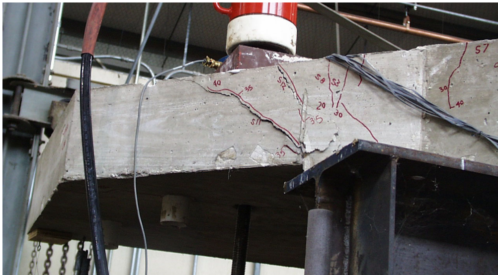
Figure 6-12 Failure of breakback IBTS overhang, side view, facing northeast
