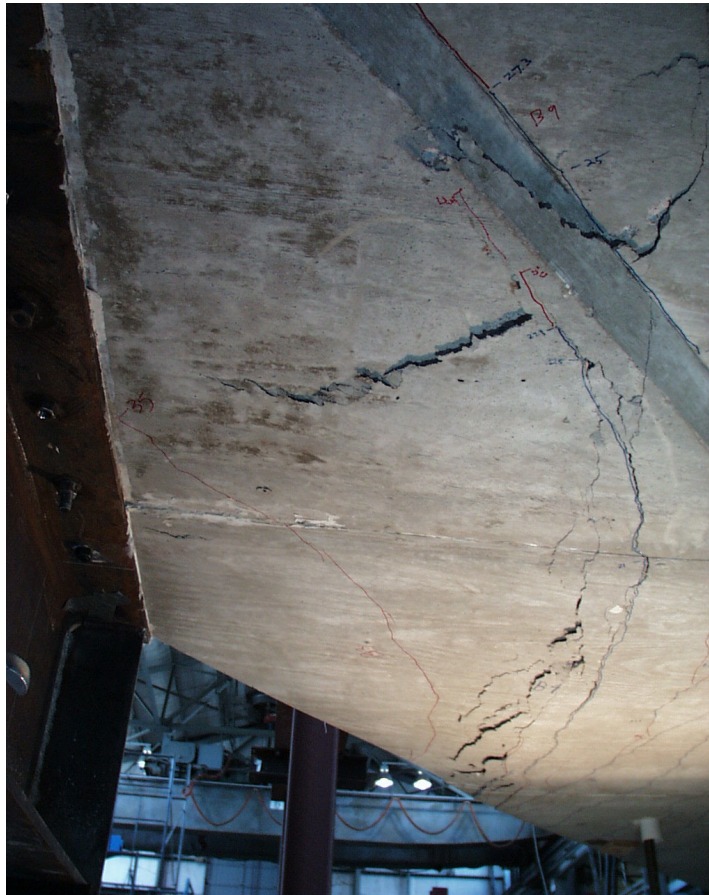
Figure 5-40 Failure surface at bottom of slab, facing south
